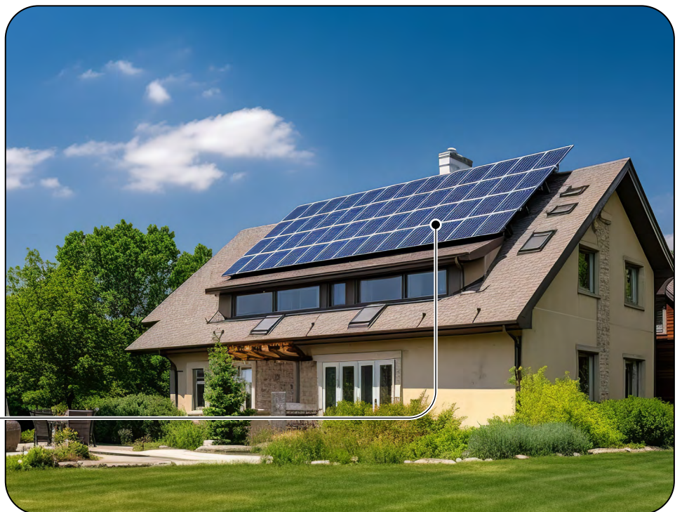
Solar panels on a home's roof turn solar energy into electricity.
