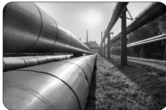
Pipelines are used to transport propane and natural gas to a processing facility.
