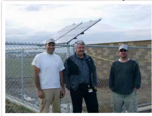
Following installation of the PV system, Bret Sutterley (center) discussed the project with the contractors, Brad Price (left), owner of Valley Solar, and one of his employees.
